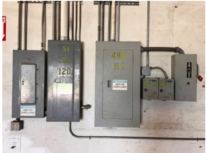
Heavy Power (3-Phase, 800a, 480v)
