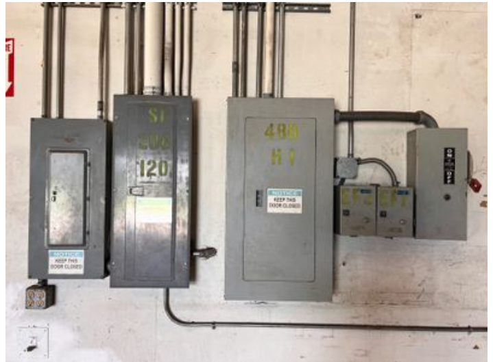
Heavy Power (3-Phase, 800a, 480v)
