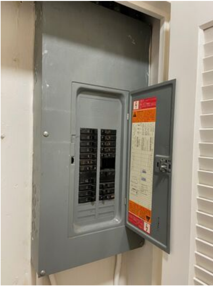
Office Electric Service
